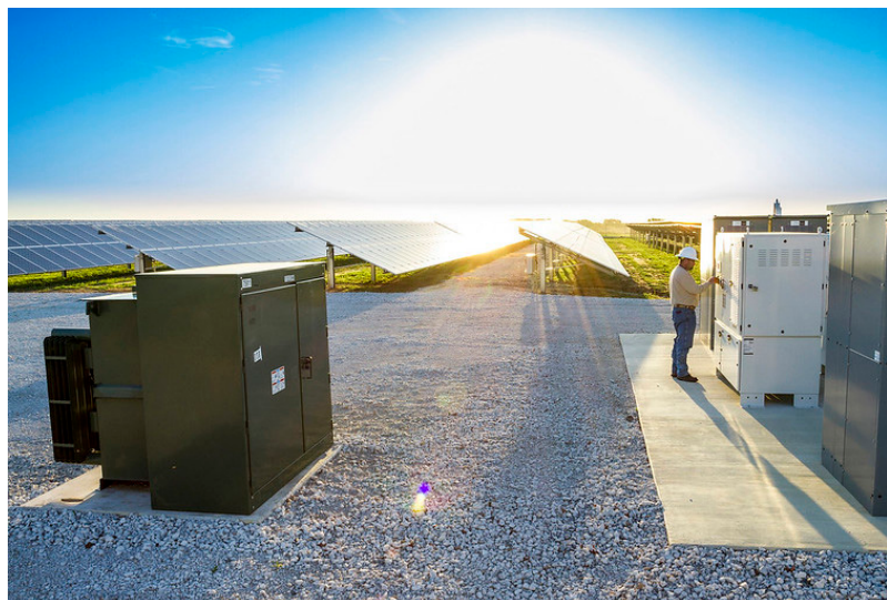
A worker checks on an inverter at a large power plant. Photo by Ken Oltmann/CoServ.
